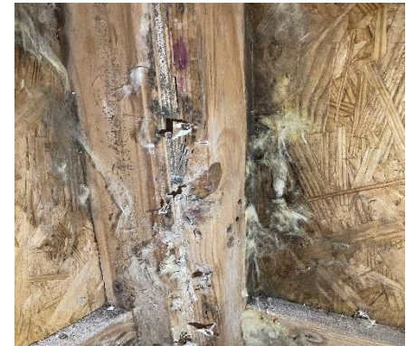
Mold inside a wall cavity
