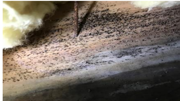
Mold on crawlspace floor joist
