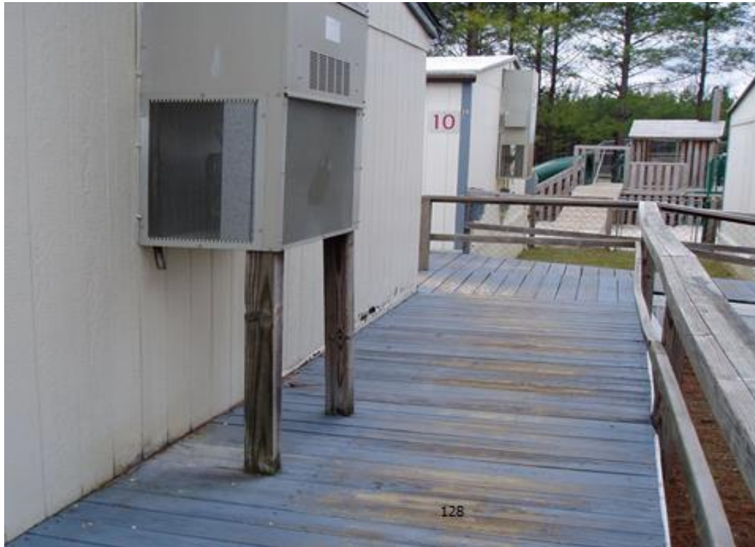
Poor condensate drainage
