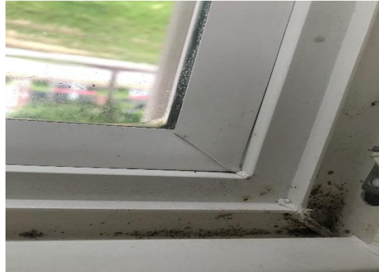
Mold on windowsill
