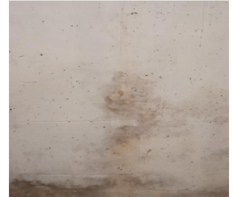
Mold growth in drywall
